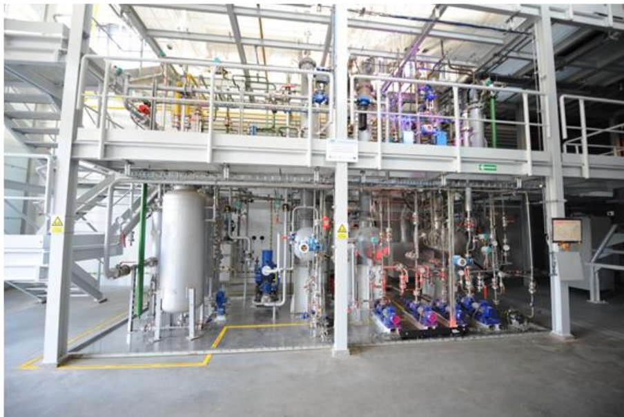
Fig. 1: Overview of the PDU for amine-based post-combustion carbon capture at Clean Coal Technologies Centre in Zabrze, Poland.
